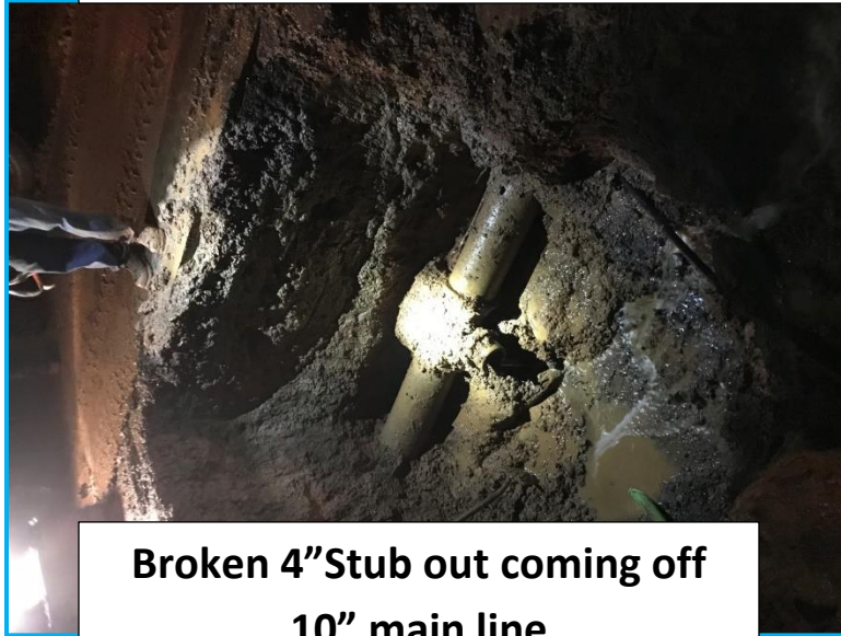
Water Flooding Pine MTN. Drive Left Broken 4" stub out Right
