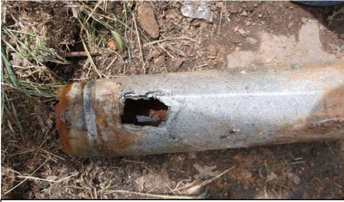
Deteriorating water pipe causing water break
