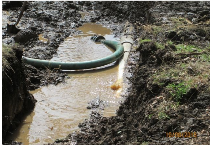
Water break resulting from weak and deteriorating aging distribution system
